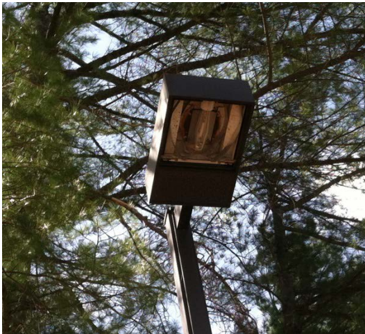
Yard lighting before project
