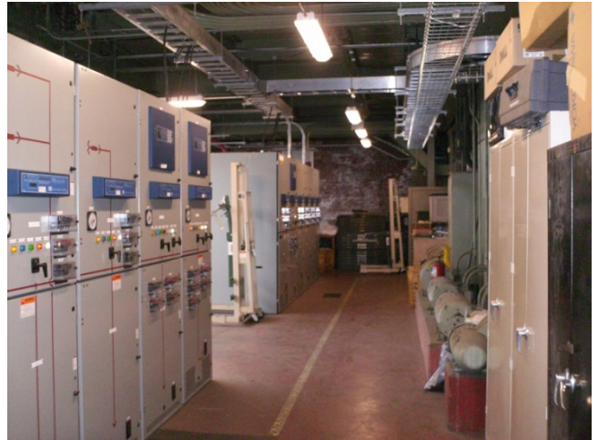
Motor control area after project
